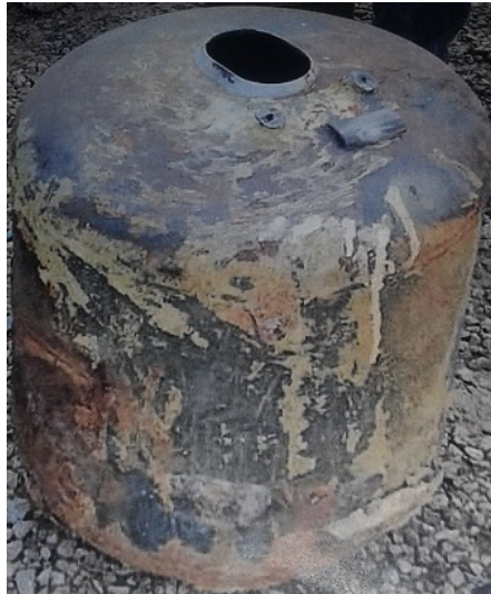
Figure 1: a consumed water heater
